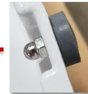
BIN SWITCH: MAGNET ON WATER CURTAIN. SWITCH IN CONTROL BOX.
